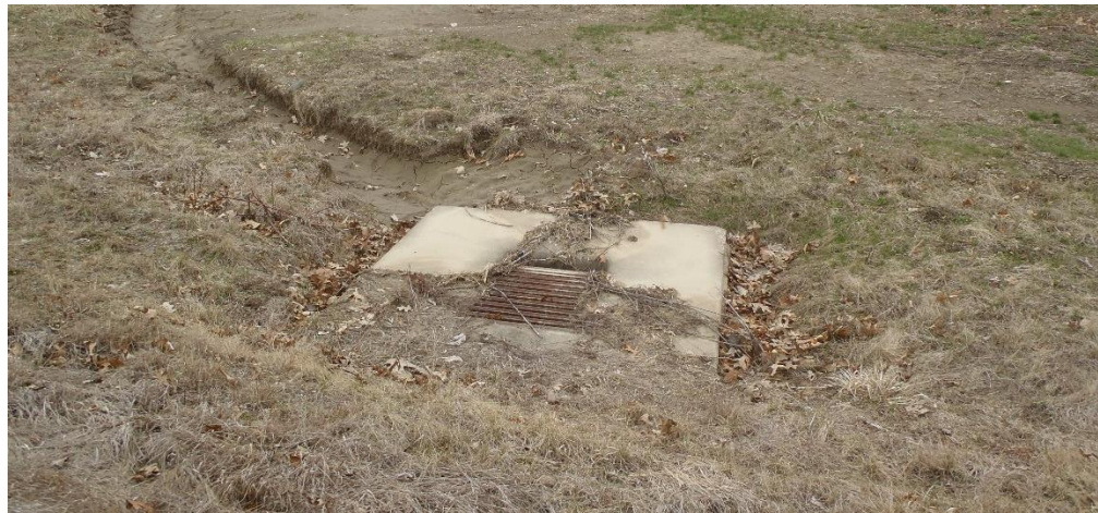
Stormwater drain needing repair and upgrading. North Hadley.
