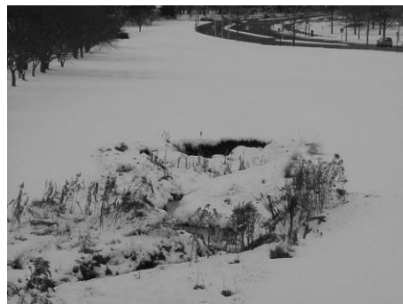
9) Keep an eye on the culvert under Mullins Way where rock used in rip rap has collected in the bottom of the culvert.
