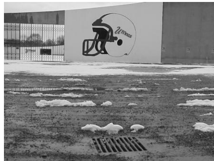
4) Source of discolored water discovered just south of Alumni Stadium where storm drain receives the runoff from a trap rock parking lot.
